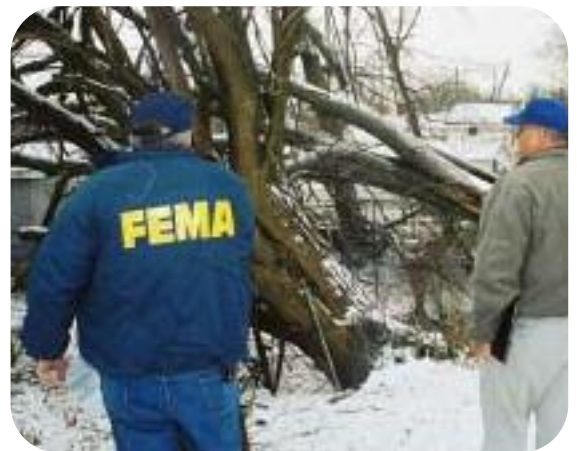
Lexington, KY, March 18, 2003 – Damage assessment teams from Kentucky’s Division of Emergency Management, and FEMA look at a tree that fell on a home in Lexington. President Bush declared 51 Kentucky counties federal disaster areas -Jason Pack/FEMA News
