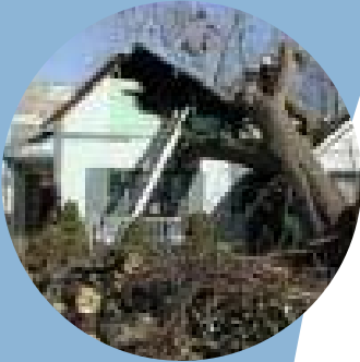
Independence, MO, February 8, 2002 – The ice has melted, but the resulting damage remains. Ice covered the tree that fell through the roof. Photo by Dave Saville/FEMA News
